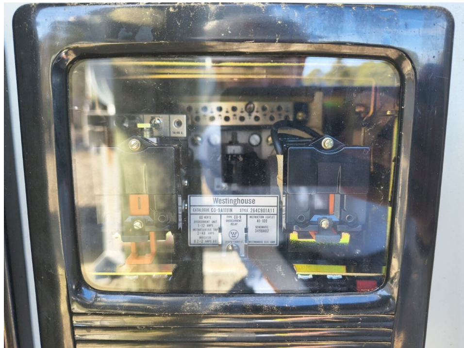
Photo 5: Electromechanical relay at Highway 71 Substation
